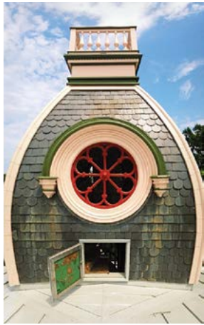
Rear of tower as seen from roof. Access hatch can be seen open at bottom. The widow's walk is the small area at the very top of the tower surrounded by a low balustrade. It has been told that the wives of seamen would watch for the return of their spouse's ships from this vantage point on coastal houses. All too often, the sailors were claimed by the sea, leading to the term "widow's walk."
