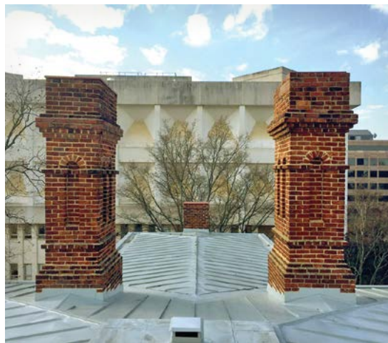
The two remaining chimneys. View looking toward rear of the house from a roof access hatch in the tower.
