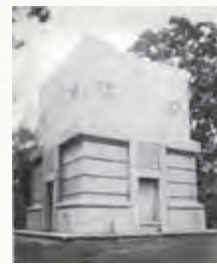
The first phase of the Memorial Bell Tower, its base, is complete, 1924.
