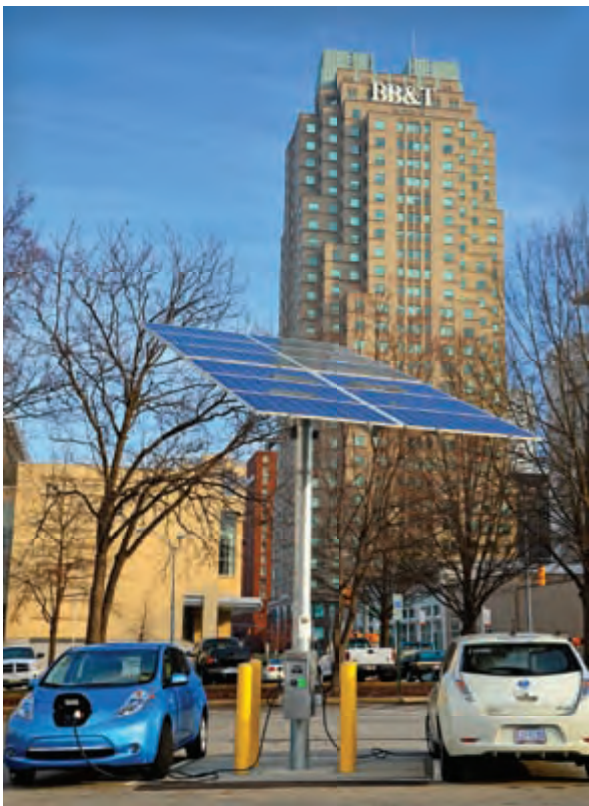
Solar-powered electric vehicle charging station in downtown. BY STAFF PHOTOGRAPHER THOMAS M. WAY
