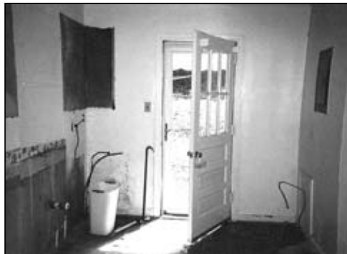
The kitchen with the appliances and counters removed
